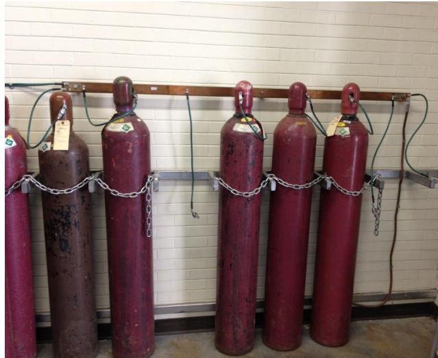
Figure 8: Compressed gas cylinder storage area. Image courtesy of WSEP.
