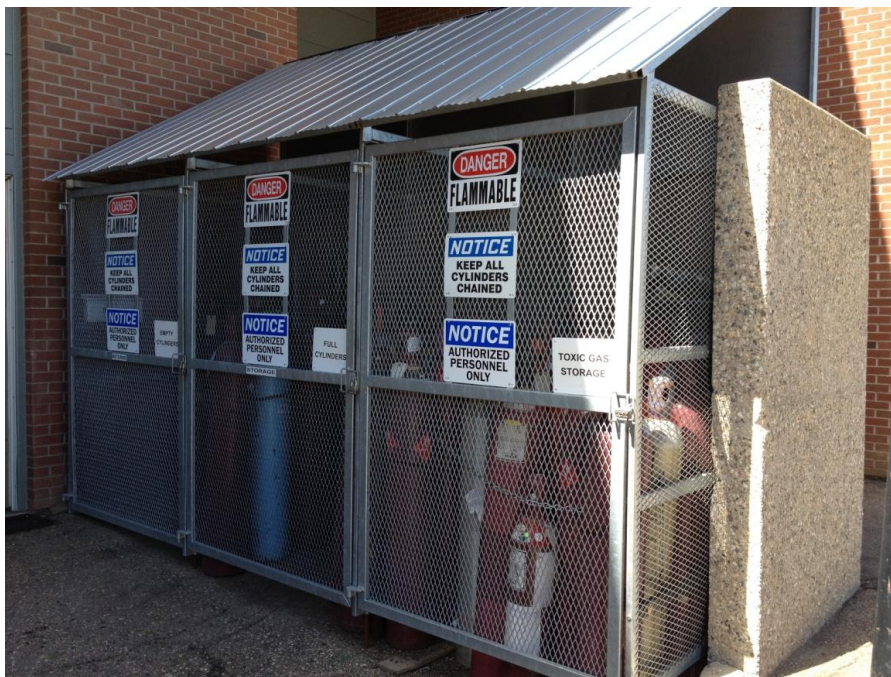
Figure 10: Outdoor cylinder storage facility. Image courtesy of WSEP.
